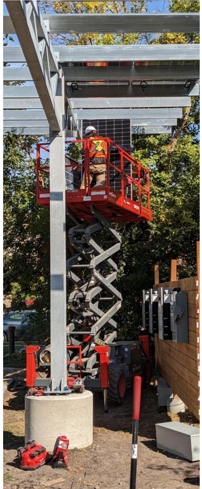
Lakeview Village Beneficial Electrification and Solar + Storage Project
