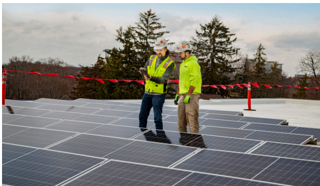
Three solar arrays were installed last year on Findorff facilities.
